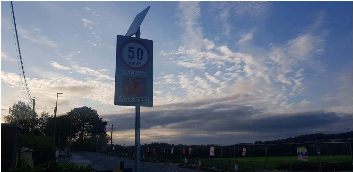
Figure 4: VMS south of CWRR Junction
